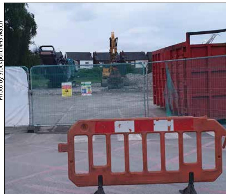
Demolition site that used to be an Outpatients at Stepping Hill Hospital.
